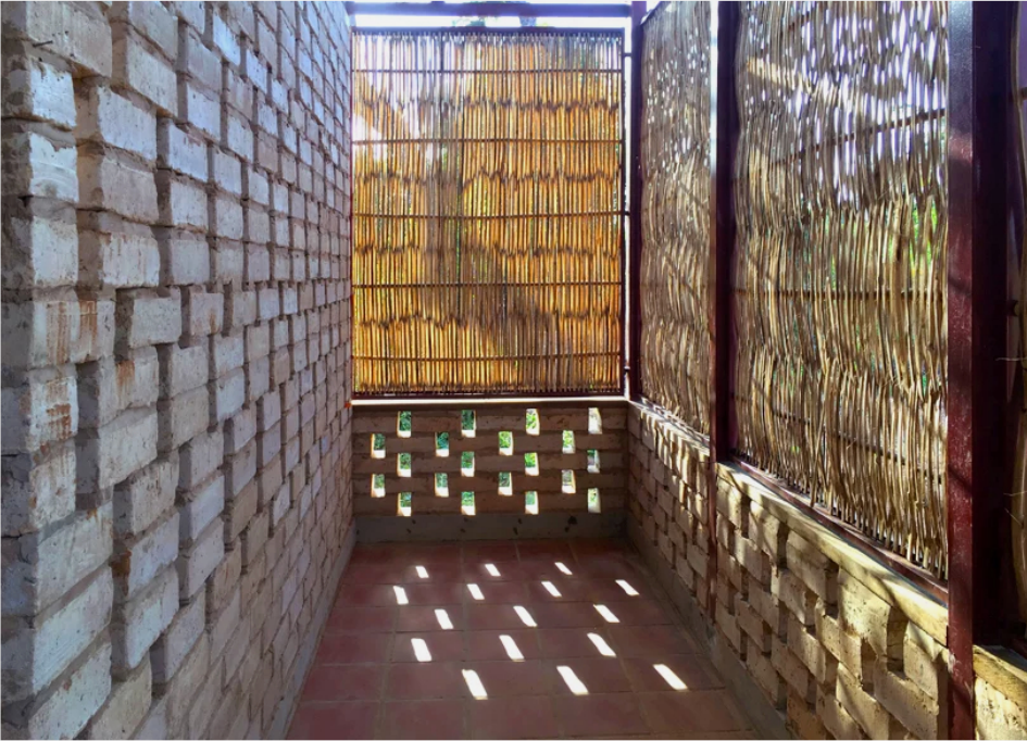
a latticed brick pattern combined with woven bamboo screens provides shading from the sun and ventilation
